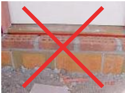
1. incorrect Kordon TB installation. Refer kd 001 and product design principle
