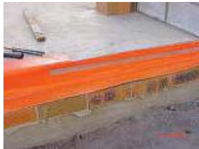
4. if tiling is to extend to slab edge Kordon TB is installed as shown - secured with gal hoop-iron/strapping.
